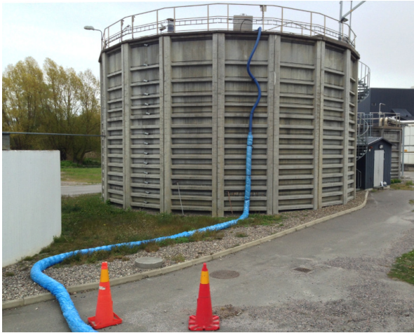
Figure 4.4. The SBR at Slotshagen WWTP and the temporarily installed pipe for pumping RAS to the SBR.
