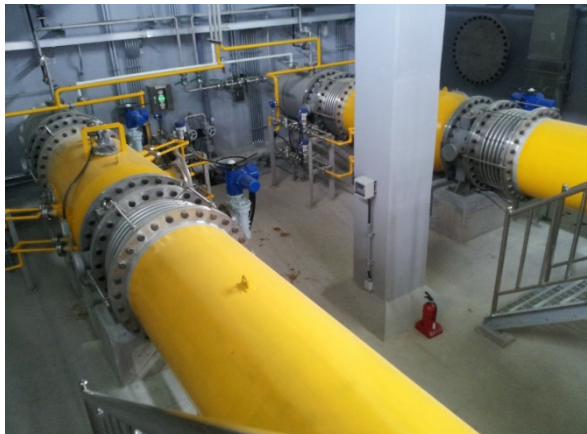
Figure 11 A full-scale installation of static mixers in the main flow pipes in a potable water plant in South Korea. Photo by PAOR CO., Ltd. (reproduced with permission).
