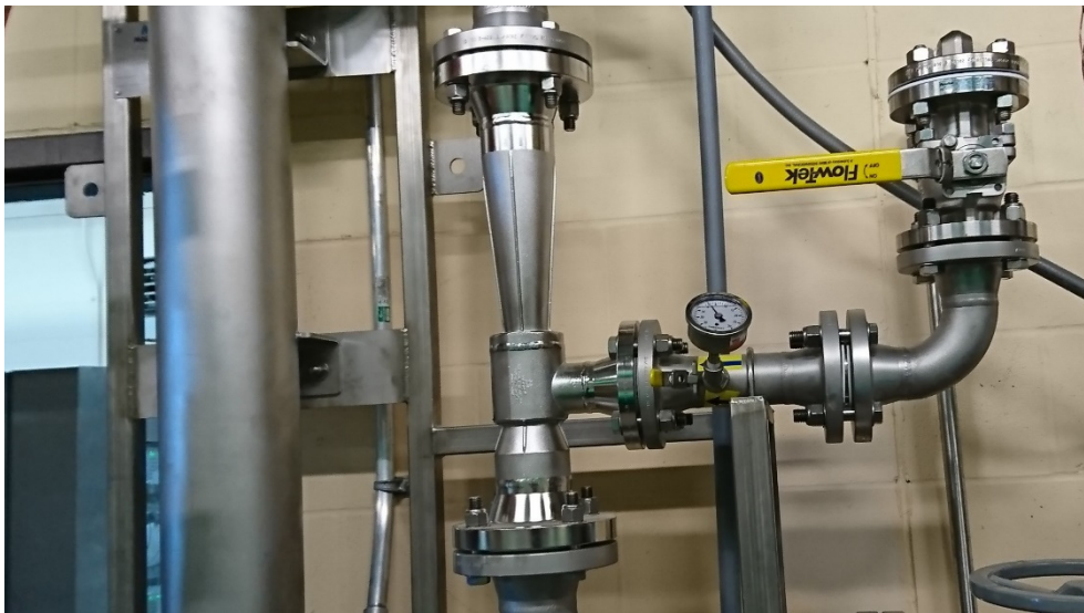
Figure 9 A venturi injector installed at a potable water plant in the US. The water flows upwards and ozone is injected in the port on the right hand side. Photo by Mats Cato (reproduced with permission).
