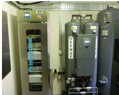
Figure 2 Inside view of the same container. Visible from the left - main PLC, ozone generator, and oxygen generator.
