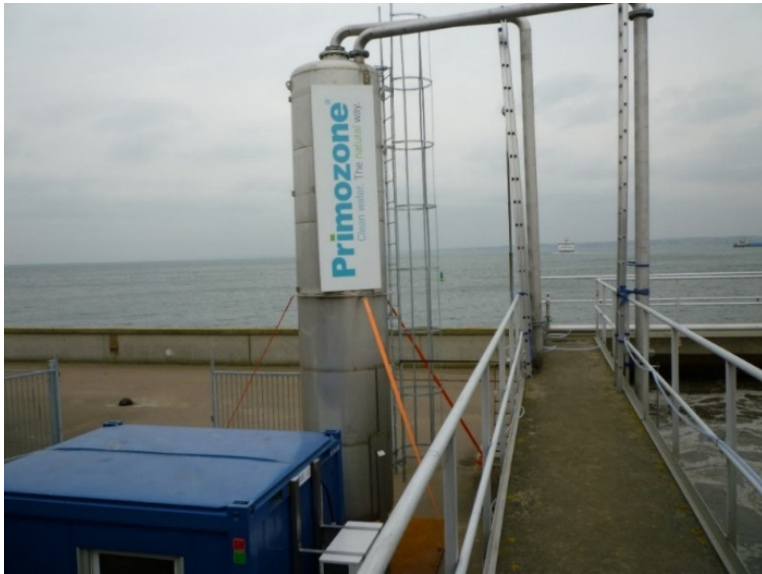
Figure 4 Picture of the container and pressurized reaction vessel installed at Öresundsverket WWTP.
