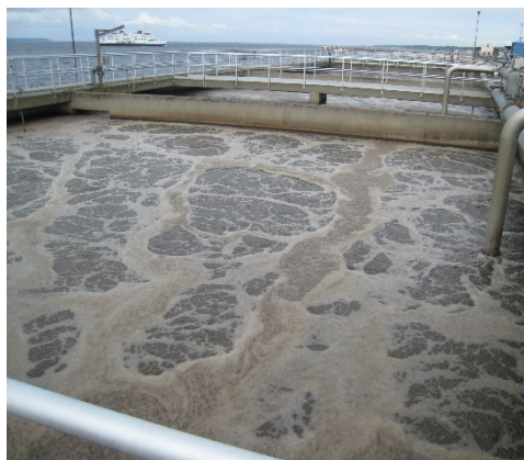
Figure 25 Aerated zone of ozone treated line at Öresundsverket WWTP.
