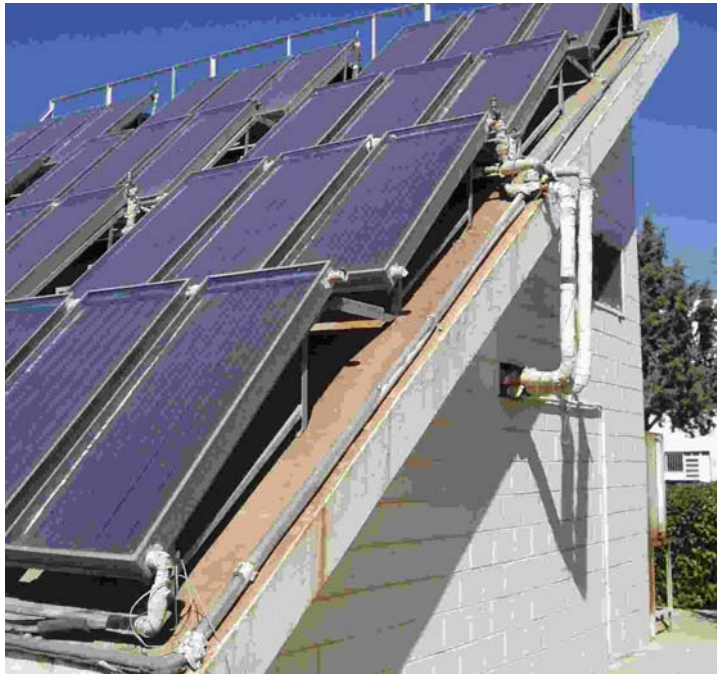
Fig. 4.1.8 Photo of the existing large system flat plate collectors at the RSS.
