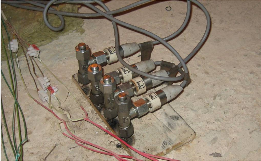
Figure 23 The pressure gauges and the T-junctions used in the pressure measurement system.
