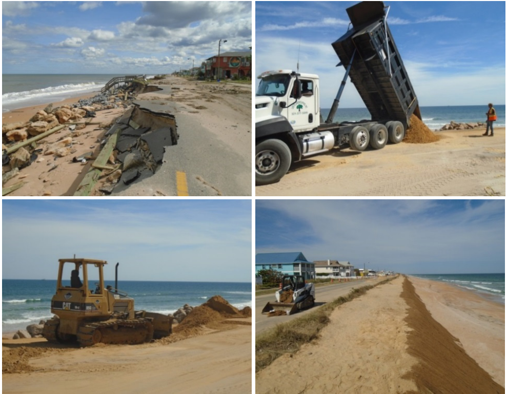
Figure 26: Top left: Damage to SR A1A post-Hurricane Matthew. Top right: Dump trucks haul loads of sand during reconstruction of SR A1A. Bottom left: Bulldozers spread fill sand and grade the newly constructed road side. Bottom right: SR A1A after reconstruction, with filled and rebuilt sand dune covered with burlap fabric (and eventually with rocks).
