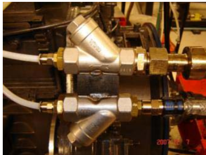
Figure 46 Pressurized air switching system built up by two check-valves.
