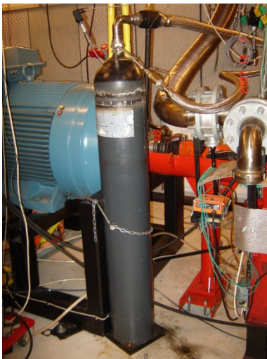
Figure 5 The pressure tank connected to the cylinder head by metal tubing
