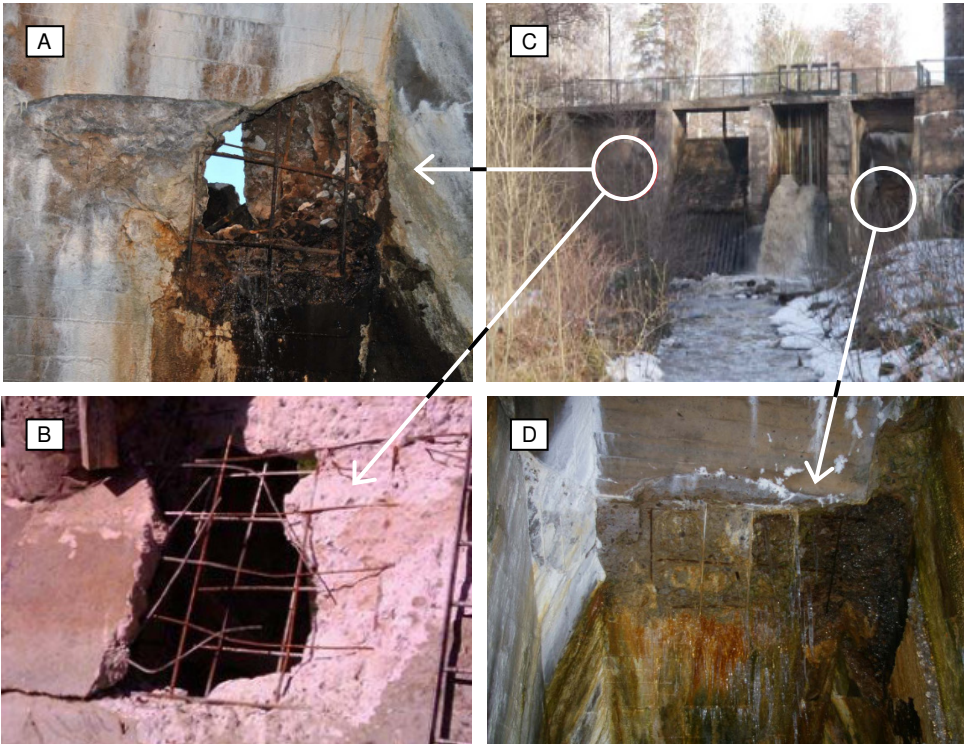
Figure 3-3. A severely damaged buttress dam (C). The concrete cover was missing in some places in the vicinity of water leakage through cracks on the downstream face (D). A hole appeared in the flat slab in another place and water escaped flushing away loose pieces of concrete (A-B). Only the reinforcing steel was left.
