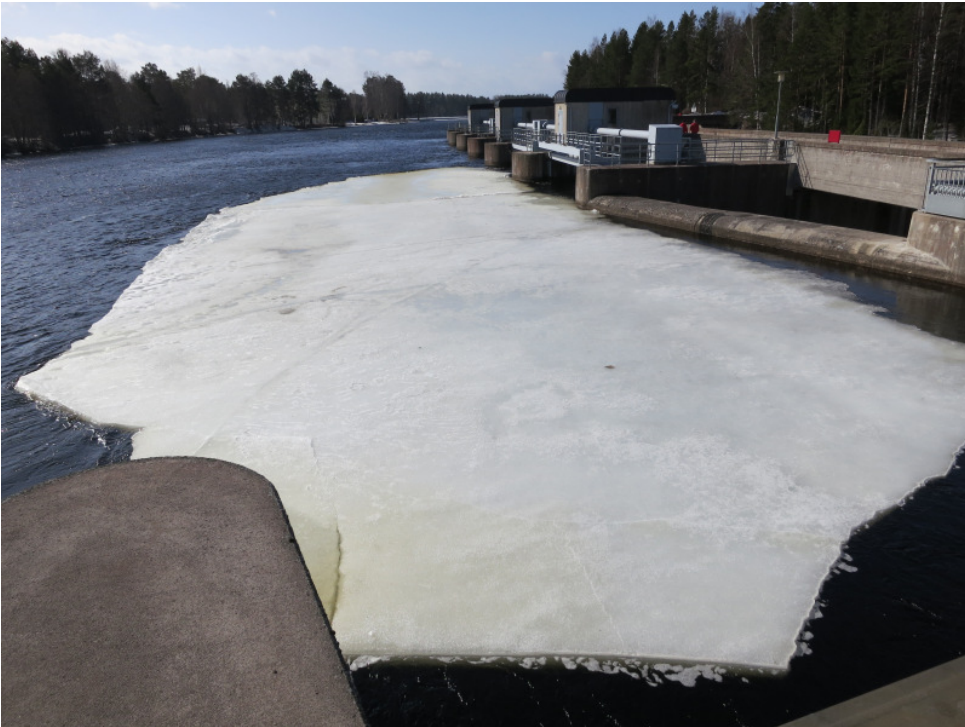
Figure 2-9. Ice floe pushing against a bridge column in spring.
