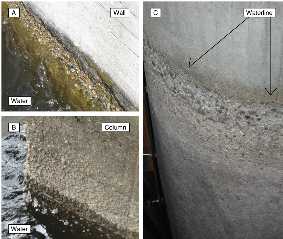
Figure 3-1. Photos of damage to the concrete surface at the waterline of hydro power structures. The photos A and C are taken on the upstream side, whereas the photo B is taken on the downstream side of the dams.
