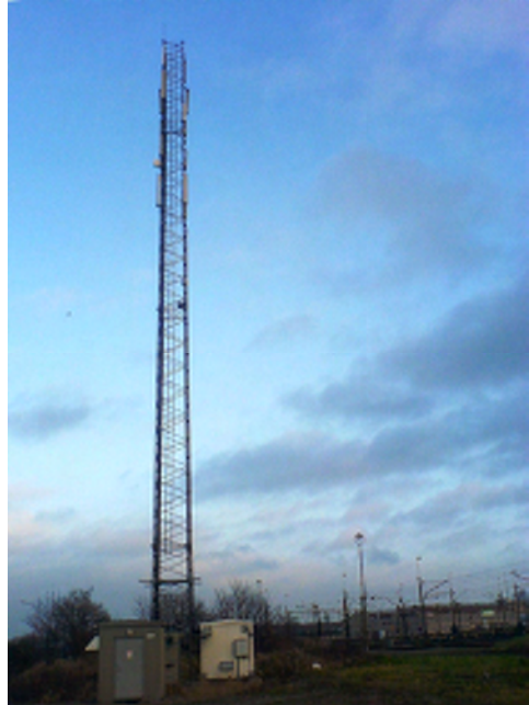
Mast in Malmö shared by Svenska UMTS (Telia Sonera/tele2) – using it for both GSM and UMTS, Vodafone (Telenor), and Tele2 – using it for GSM.
