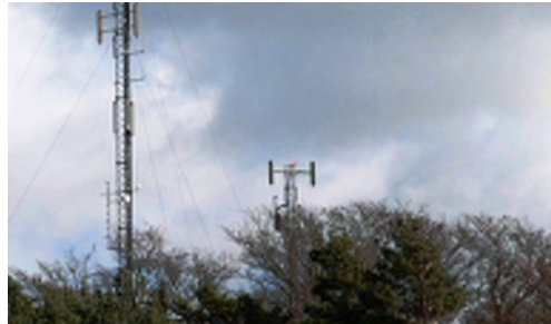
Picture: Double masts southeast of Sjöbo, Sweden. In 2001 and 2002 1/3 of the municipalities received mast building permit applications for masts less than 100 metres from each other.
