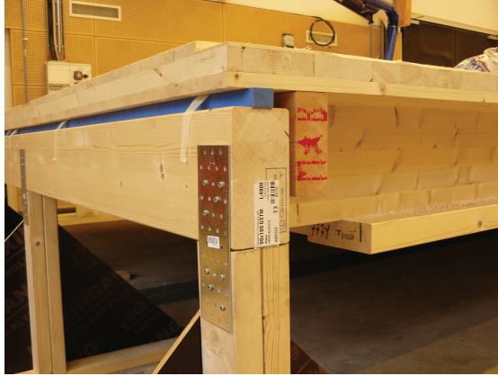
Figure 10: Floor supports joined to a glulam beam by means of a tie plate, the floor resting on top. In this case, the floor is required to rest on top of an elastomer, blue in colour in the picture, according to the manufacturer's instructions.
