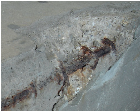
Figure 1. Severely damaged concrete, caused by corrosion of steel reinforcement bars. Original figure by MADe (licensed under CC-BY-SA-3.0)
