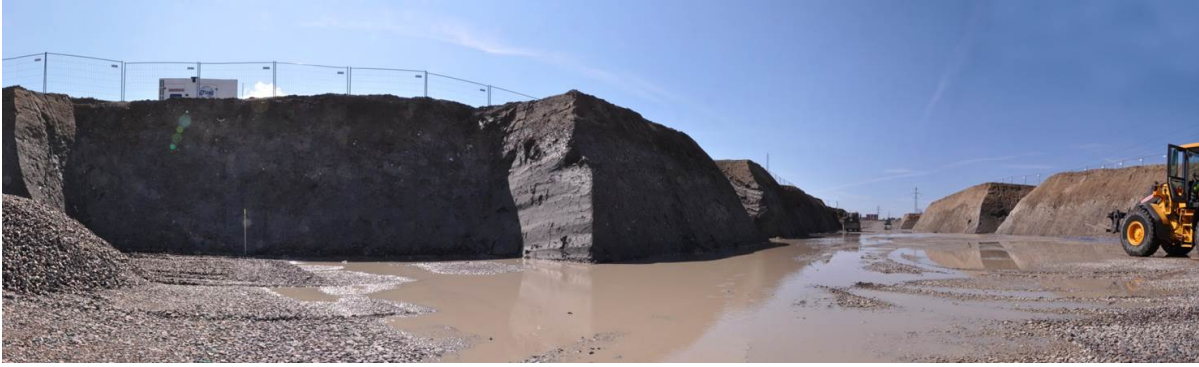
Figure 2.4: A photograph of the soils at the excavation site for the Linac tunnel.
