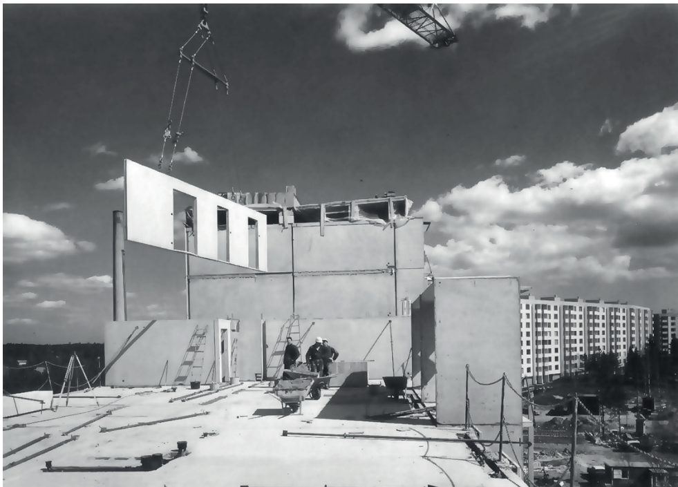
Figure 4 Assembly of prefabricated wall elements in a house-building project in the Million Homes Programme (Marmstål and Nordberg, 1992).
