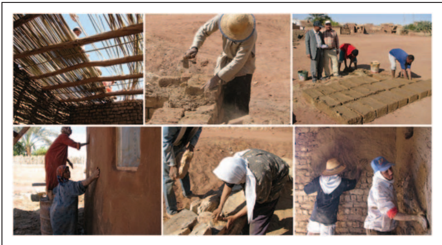
Figure 11. The built room of the neo-desert vernacular model house during different work phases.
