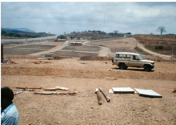
Figure 4. A view of the site before self-construction. Photo: Arturo Robles, project architect
