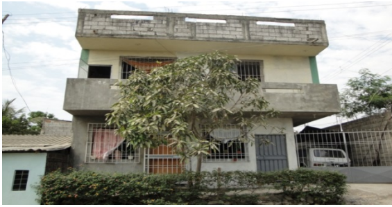
Figure 9. New housing replacing second housing typology in phase 7 with reinforced concrete structure and masonry block walls. Photo: Ivette Arroyo, 2009
