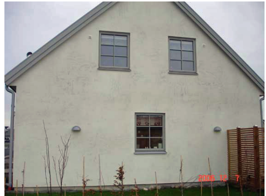
(b) Building with mould growth
