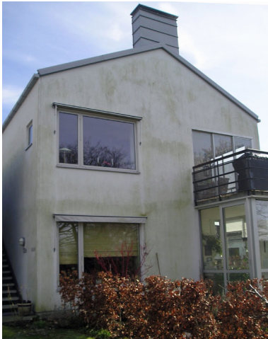
(a) Building with algae growth
