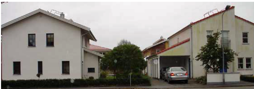
Figure 2.3: Two neighboring houses in southernmost part of Sweden. The house to the left has no discolorations whereas the house to the right have pronounced discolorations due to algae growth.
