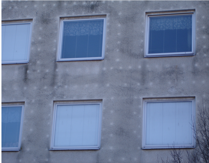
Figure 2.8: Another façade with white spots.
