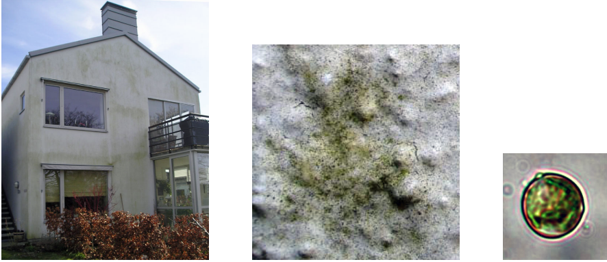
Figure 3.1: Algae growth on a building façade (left), a close up picture (middle) and as seen in microscope (x400) (right).
