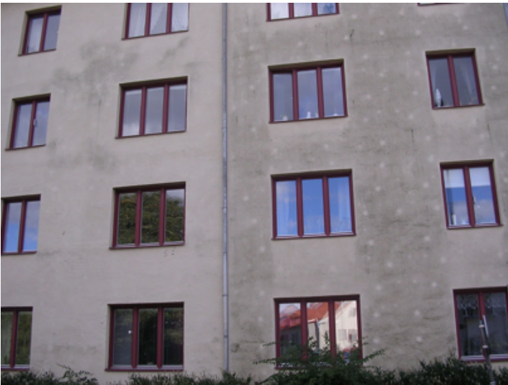
Figure 2.7: A façade that shows white spots.
