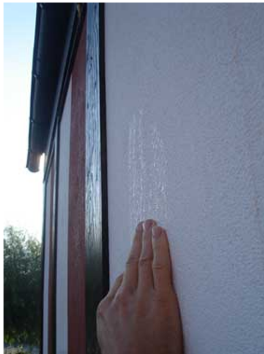
Figure 2.11: Night condensation of a north-facing wall on the test house (Paper III) around 8 in the morning in October 2007. No condensation was found on the south-facing façades or on the walls with render on bricks.
