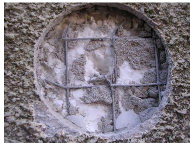
(b) Below the gray part of the façade without the fastener
