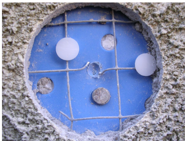
(a) Fastener below the white spot on the façade
