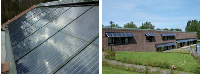
Figure 1.6 Left, building integrated PV modules. Right, PV modules working as a sunshade. Thanks to GAIA Solar for photographs.
