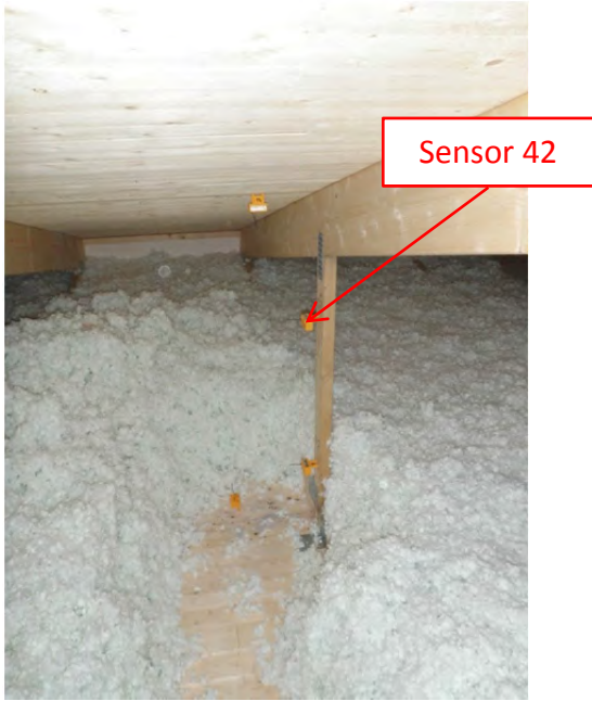
Figure 9.42.5. Location of the studied position. The cellulose fiber insulation was temporary removed.
