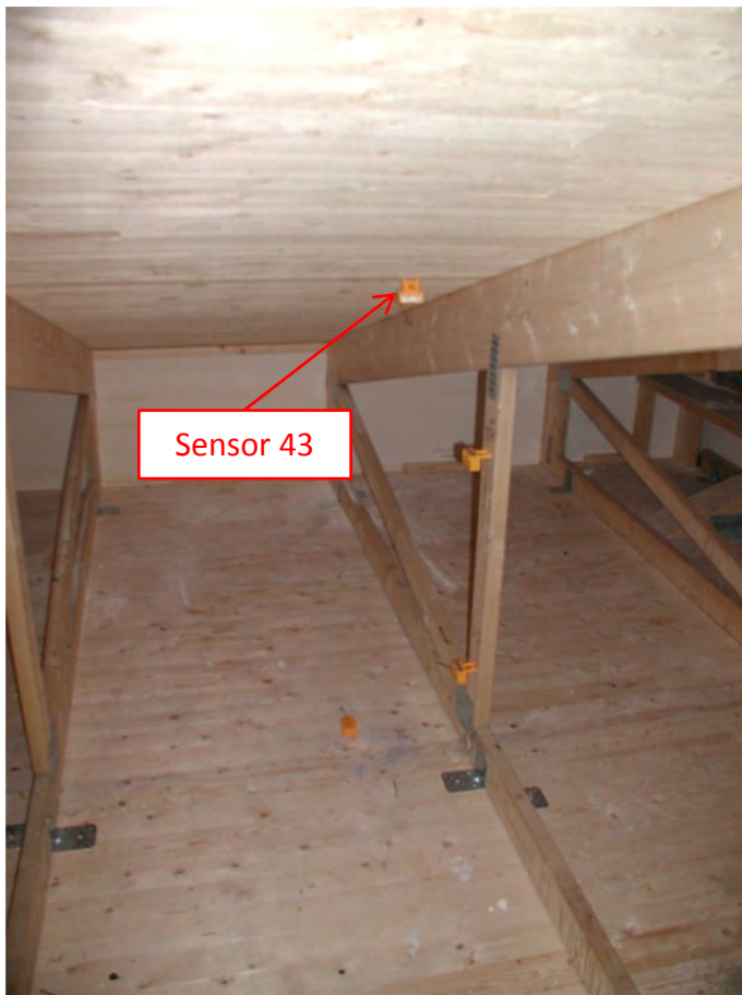
Figure 9.43.4. Location of the studied position before the cellulose fiber insulation was applied.
