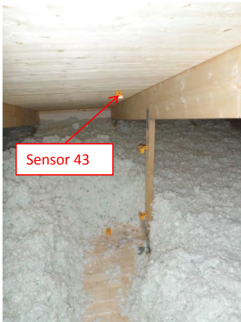
Figure 9.43.5. Location of the studied position. The cellulose fiber insulation was temporary removed.
