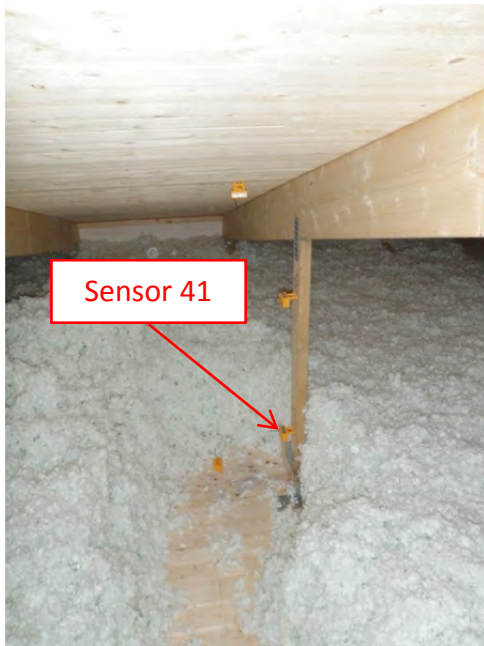
Figure 9.41.4. Location of the studied position. The cellulose fiber insulation was temporarily removed.
