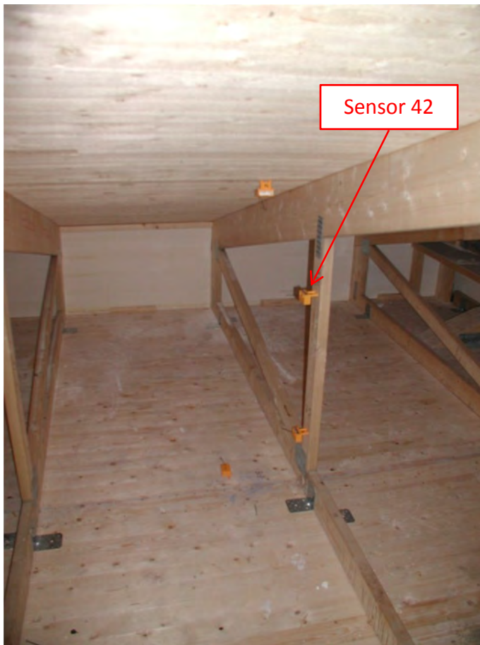
Figure 9.42.4. Location of the studied position before the cellulose fiber insulation was applied.
