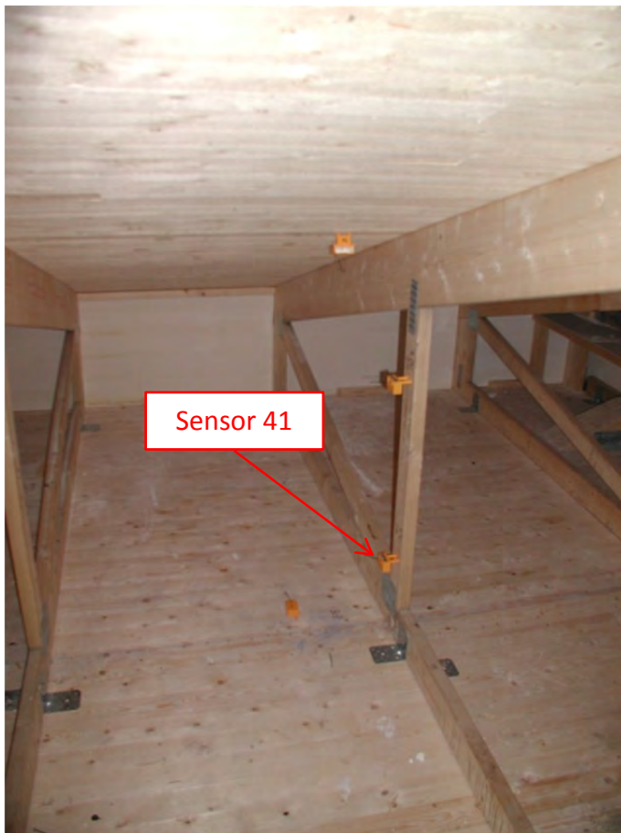
Figure 9.41.4. Location of the studied position before the cellulose fiber insulation was applied.
