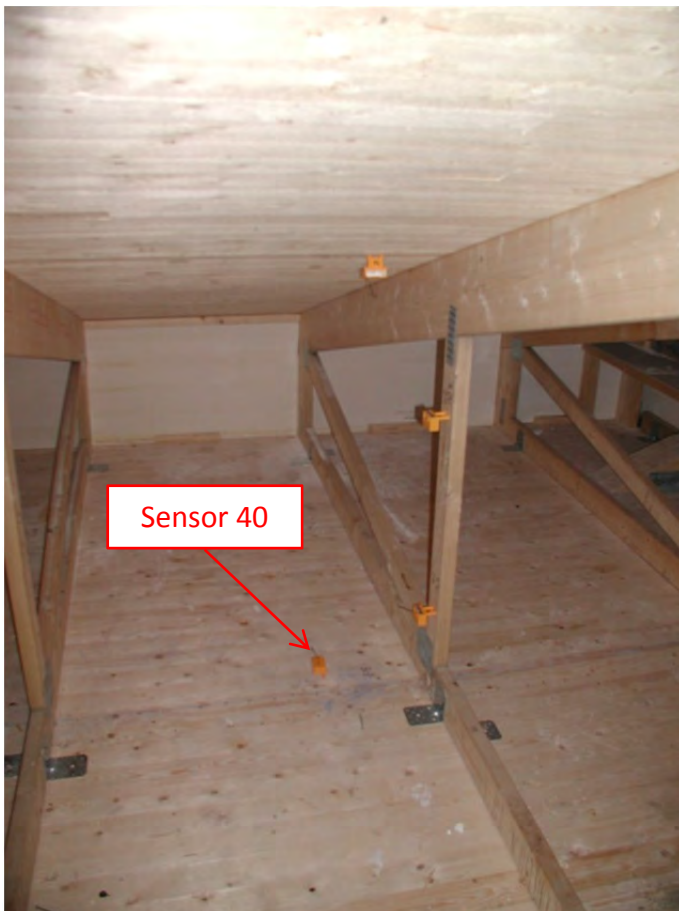
Figure 9.40.4. Location of the studied position before the cellulose fiber insulation was applied.
