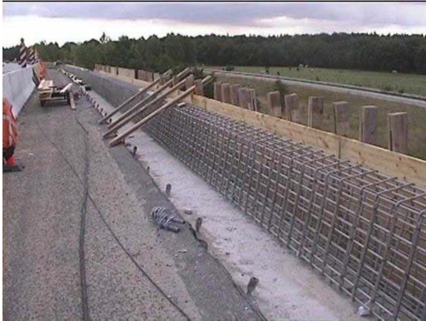
Figure 2: Repair of damaged bridge due to chloride initiated corrosion. Stainless steel reinforcement shall replace corroded carbon steel reinforcement.
