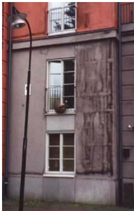
Figure 4.6 Growth of moulds on a facade
