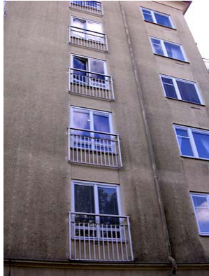
Figure 5.10 Building 3 in Kristianstad with thin rendering on thermal insulation. The grey façade is almost covered with discolorations
