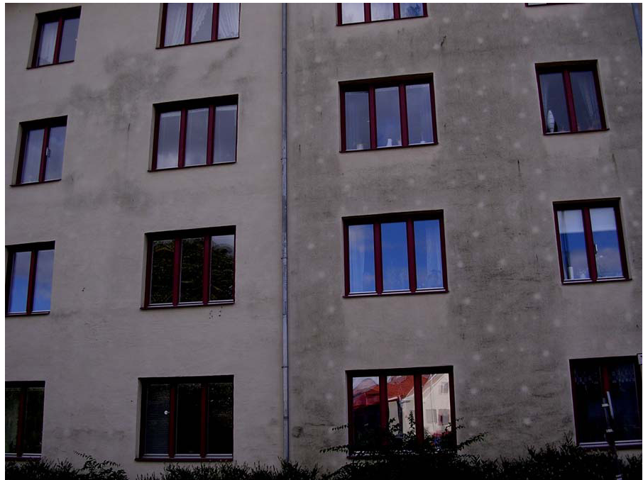
Figure 2 Façade construction with thin rendering on thermal insulation, heavily affected by microbial growth on the right part of the façade. The white dots have no biological growth
