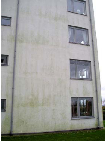
Figure 5.1 Façade of building with thin rendering on thermal insulation with green discolorations from a building in Höllviken
