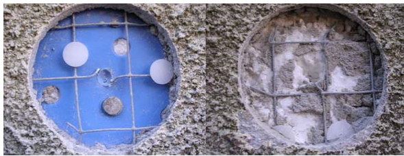
Figure 5.11 Circular holes through the rendering of the façade of building 3. Left picture shows a fastener placed under a “white dot”. The grey screw of steel holding the fastener plate is also seen. Right picture shows only thermal insulation at a place on the façade with discolorations
