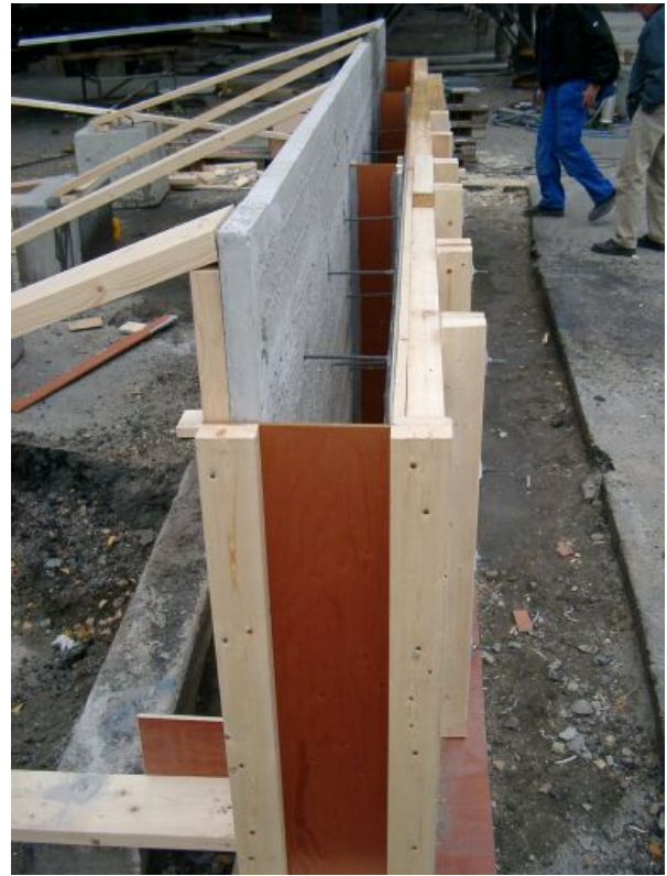
Fig. 3.5 – Field test at BTC with one side of mould consisting of a prefabricated concrete element and the other of wood or transparent glass fibre. Photo: Iad Saleh.
