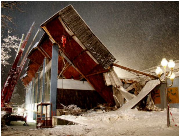
Fig. 1. Collapse of wooden roof for ice skating arena in Bad Reichenhall, Germany
