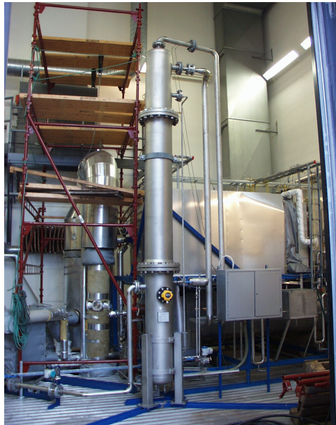
Figure 4.3: Ethanol humidification tower in the pilot plant
