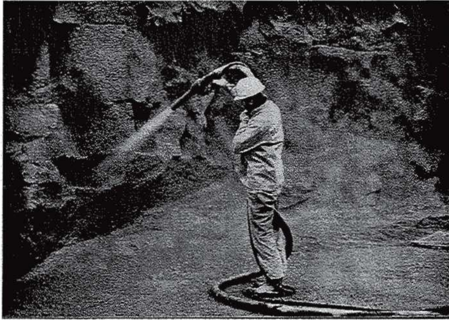
FIG 6. Fibre concrete sprayed on a an irregular rock surface allows thinner layers to be applied compared with what would have been possible with a traditional mesh reinforced sprayed concrete. (Photo: Stabilator).
