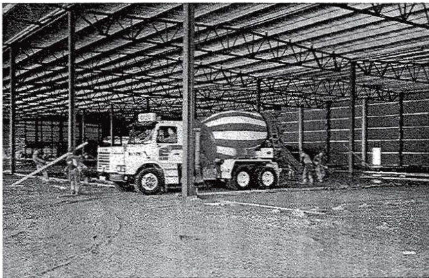
FIG 8. Producing an industrial floor in steel fibre concrete allows elimination of reinforcement placing, direct delivery from the truck and wider joint spacings.
