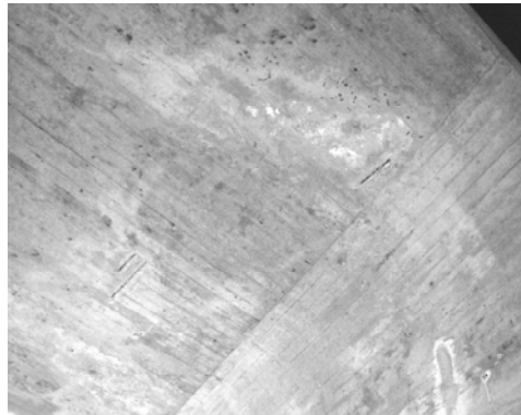
Figure B.2 Underside of trough bottom, change of colour.
