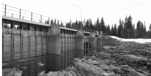
Figure 6.1 View from the upstream side of a dam, taken when the water reservoir was empty.
