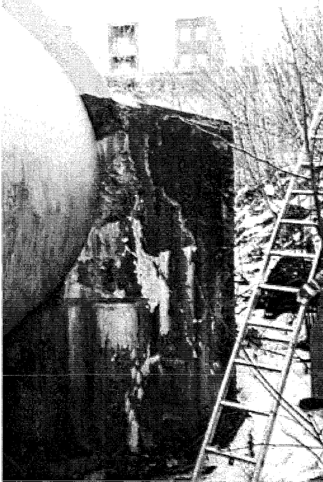
Figure 1-2 Synergy effects between lime leaching and freeze-thaw in a fix-block of concrete, supporting a water tube.
