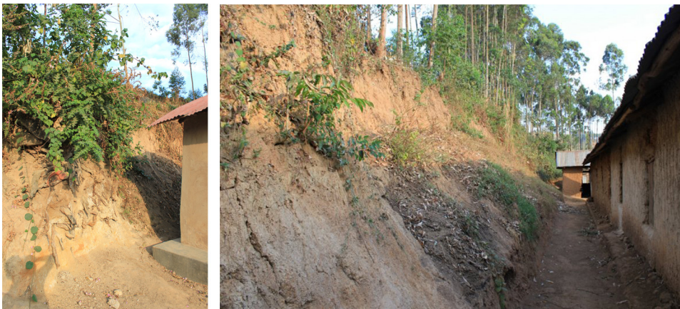
Figure 17: Photo illustrating the unstabilized slope condition behind the existing buildings
