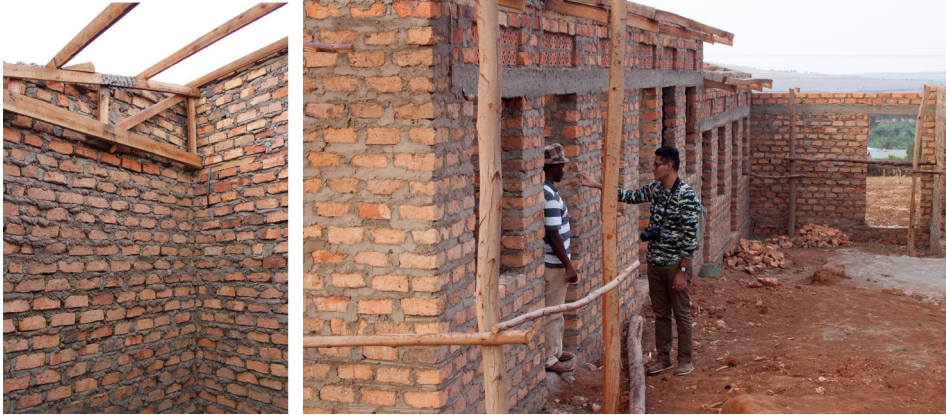
Figure 16: Pictures illustrating a typical construction site in Muhanga The pictures show a detail of the brick construction, including the various brick sizes and thickness of mortar layers
