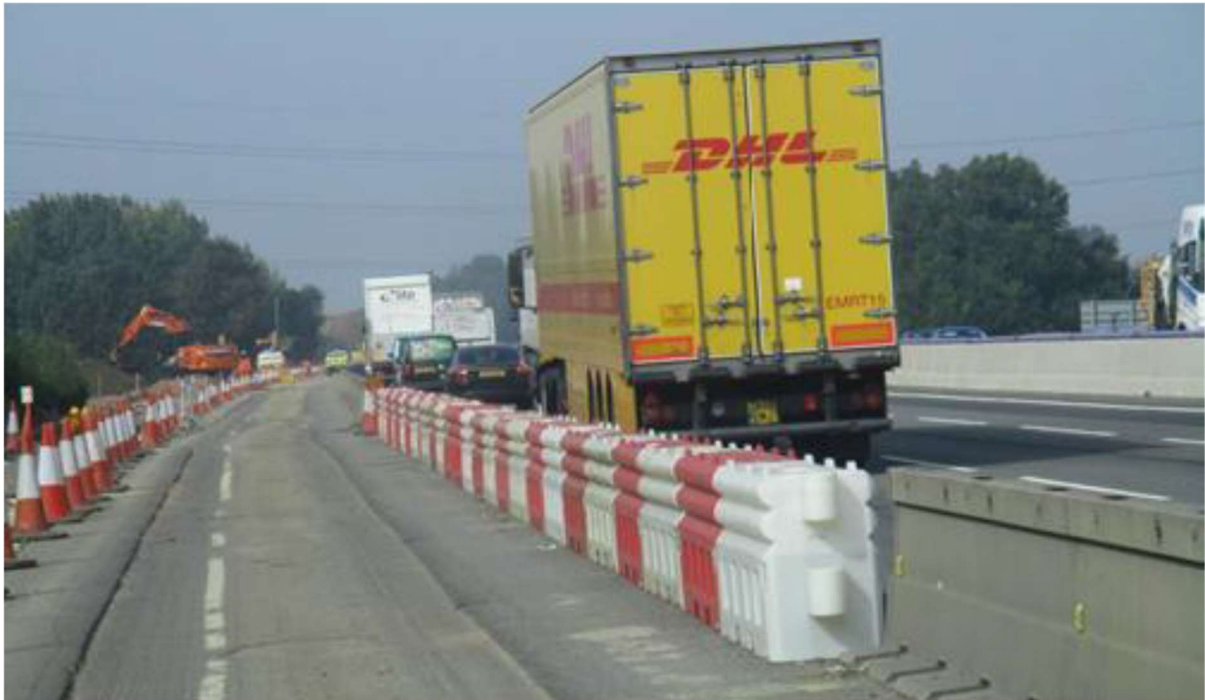
Figure 22. Water filled barriers filling the gap in the zone guard (Highway Safety Hub, 2018).
