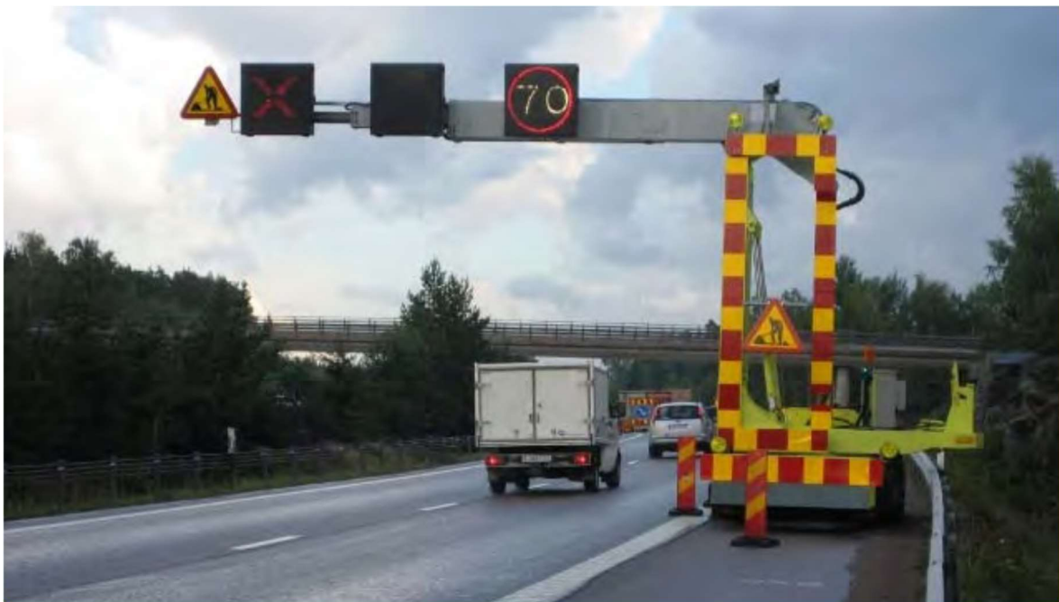
Figure 1. A mobile gantry crane for quick setup of signs at newly established road work zone (Bolling & Sørensen, 2008).
