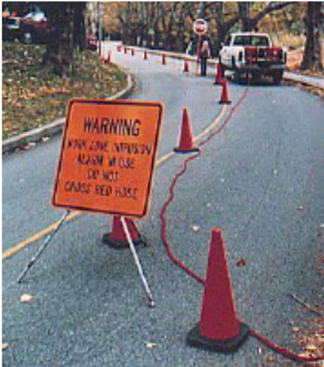
Figure 28. Pneumatic tube incursion alarm (Wang et al., 2013).
