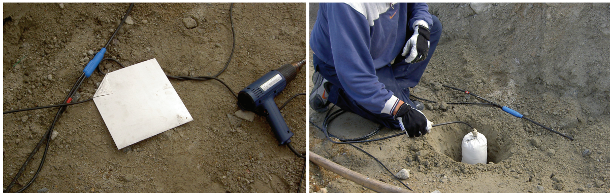
Figure 4-4 Installation of electrodes at Hällby. Left: Resistivity electrodes (steel plates). Right: Non-polarisable SP electrodes (copper-copper sulphate in bentonite-filled pre-packaged cloth bags).
