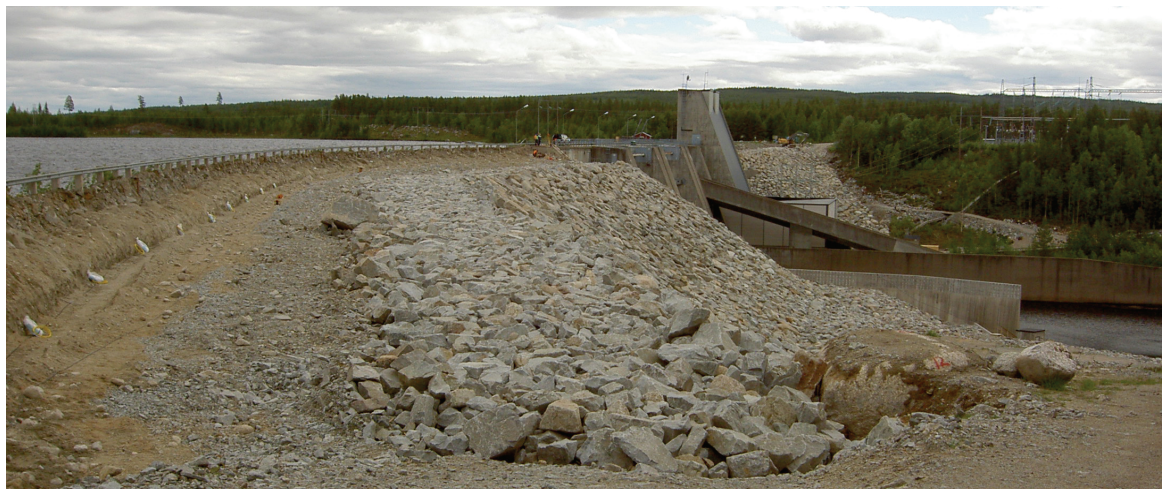
Figure 6-3 Hällby dam during the reinstillations of electrodes in 2005. The top of the right dam crest is excavated and new electrodes are being placed out, every second being a non-polarisable electrode (white bags). The downstream slope has been reinforced with additional rockfill. In the background are the spillways, the intake to the power station (high building) and the left embankment dam.
