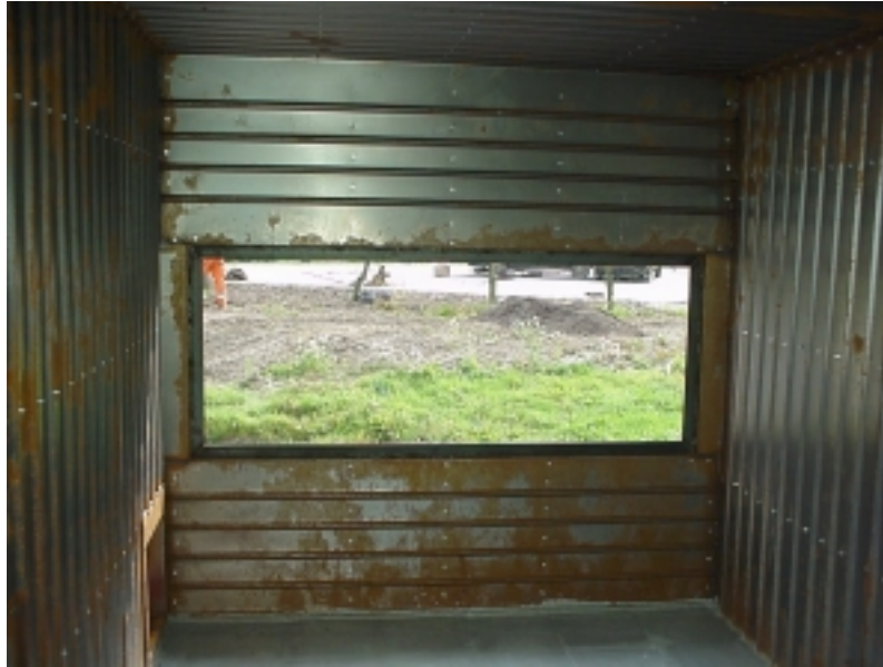
Figure 3. The opening that allows fresh air to enter the container seen from the inside.
