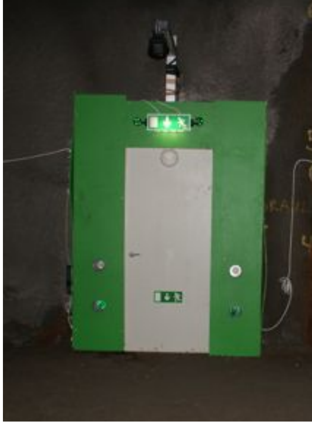
Figure 8. The emergency exit installed on the left side, approximately 180 metres into the tunnel.
