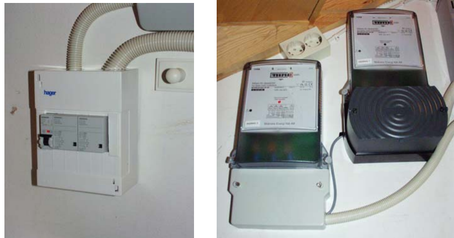
Figure 4.15. Control relay and extra meter
