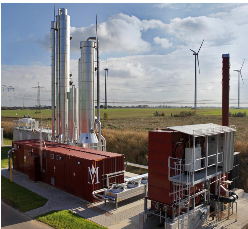
Figure 20 A water scrubber for biogas upgrading. The two towers are the absorption and desorption columns. The scrubber is equipped with an RTO unit which is shown to the right in the photograph. Image from Malmberg Water
