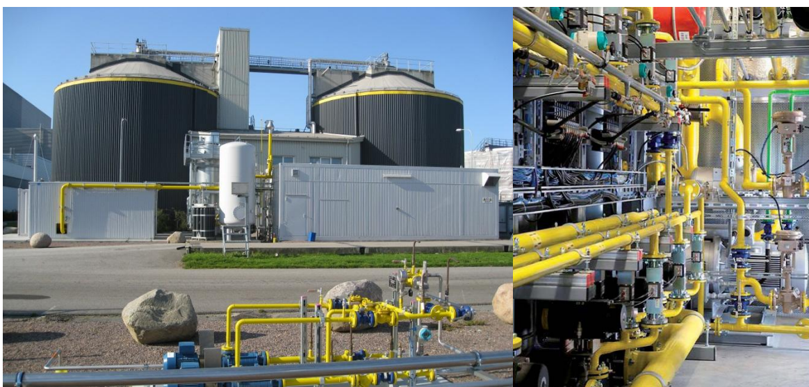
Figure 8 PSA upgrading unit in Sweden. The exterior view (left) shows, from the left, the catalytic oxidizer, active carbon filters, pressure levelization tank (white) and a container with the PSA columns. The interior view (right) shows valves and PSA columns. Images from E.ON Gas Sweden.
