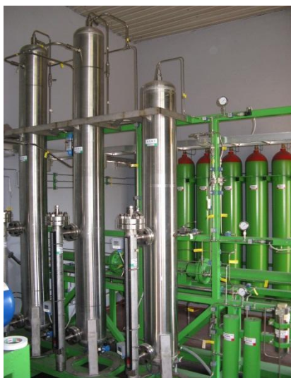
Figure 40 The columns performing the separation of carbon dioxide from the biogas in the Metener biogas upgrading system. Image from Metener Oy.
