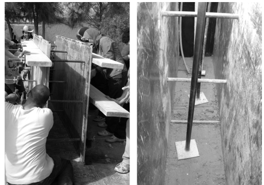
Figure 6 & 7. Left: ramming the first layer. Right: installing the formwork. Photo credit: M. Dabaieh.
