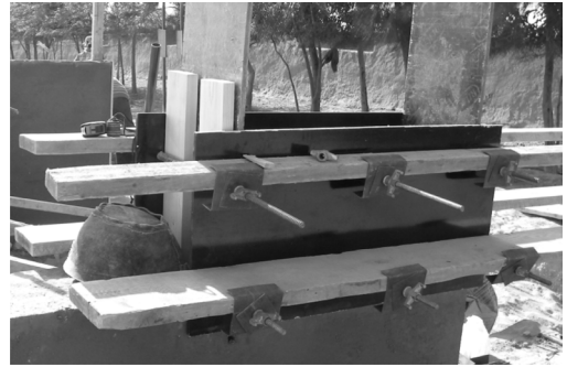
Figure 5. The formwork when assembled to ram a new layer. Photo credit: M. Dabaieh.
