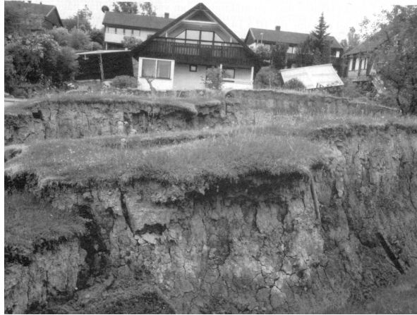
Figure 29 A photograph of a residential area in Vagnhärad after the slope failure within the Trosa River valley in 1997 (Andersson et al., 1998).
