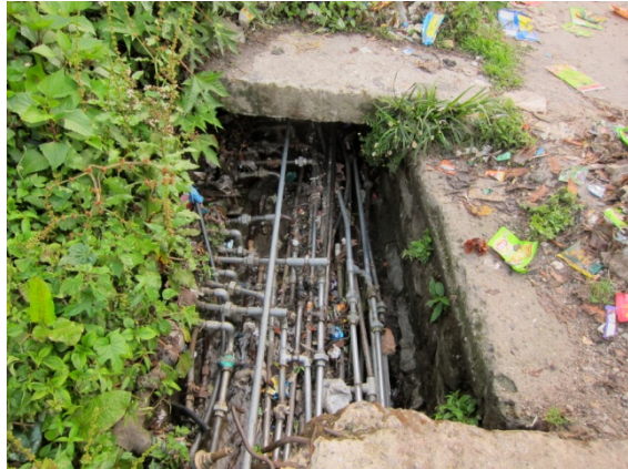
Current pipe and storm water drain infrastructure
