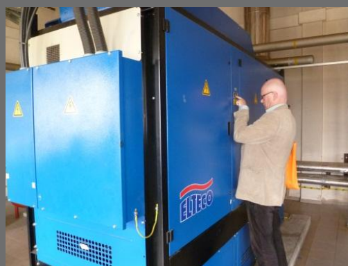
DIESEL ENGINE FOR ELECTRICITY PRODUCTION
