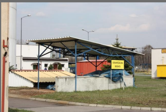
CLEANING FACILITY FOR RAW BIOGAS
