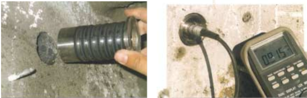
Figure 7: Mounting of proprietary corrosion sensors in existing quays. The picture to the right shows the sensor, a temporary micro-amp meter and the small titanium pin as cathode placed just above the instrument. The system is a further development from the system in Schiessl and Raupach 1992.
