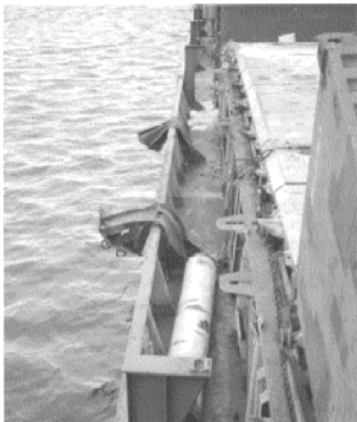
Figure 3.55: Failed deck pedestals-starboard (U.S. DOT, 1992)
