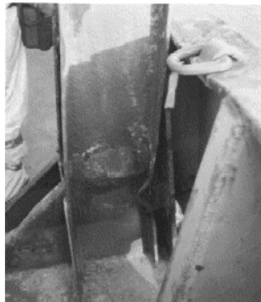
Figure 3.56: Compression damage at the bottom of pedestal (U.S. DOT, 1992)
