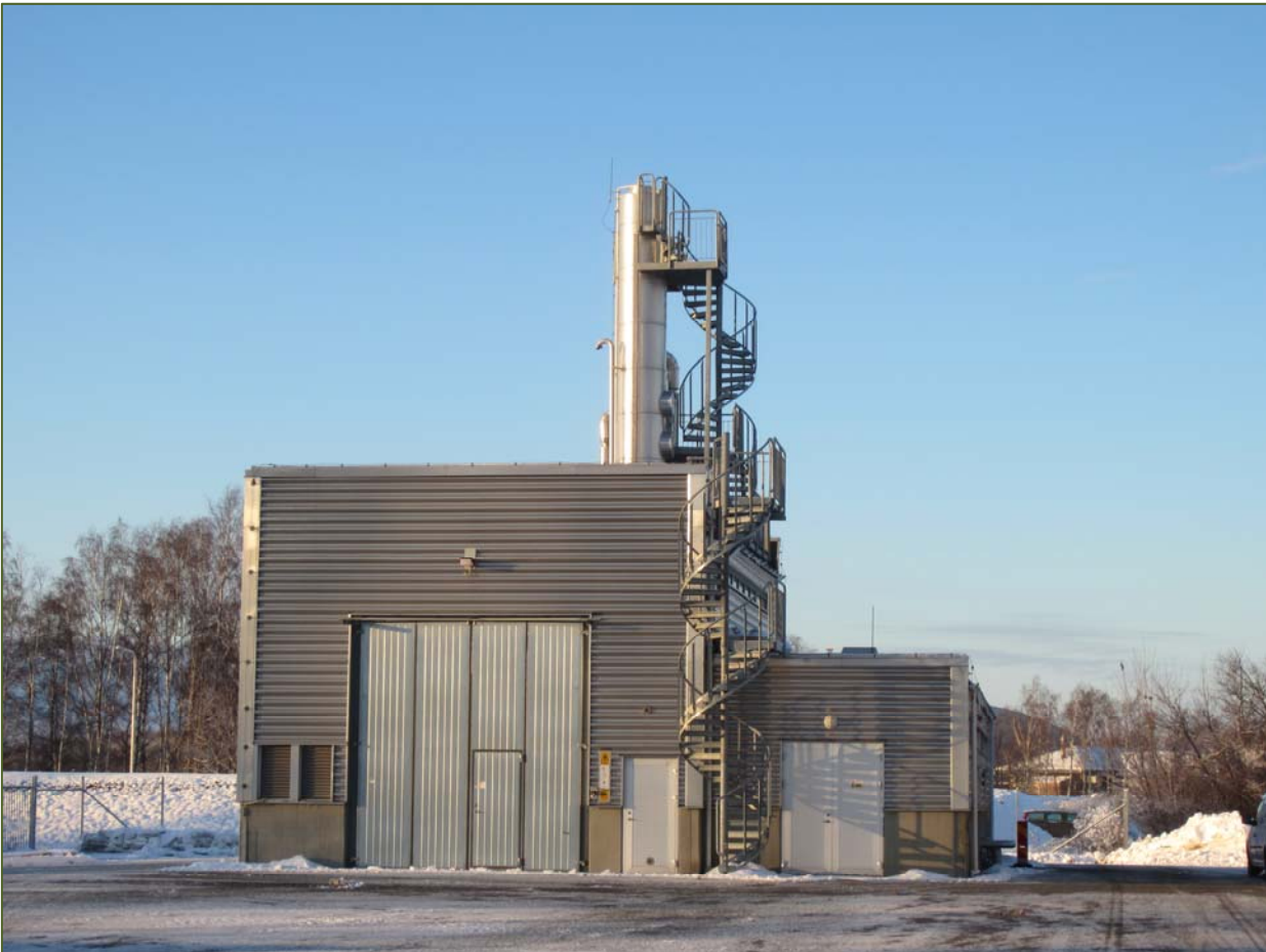
A small-scale biogas upgrading facility in Kristianstad based on the water-scrubbing technique.
