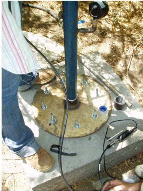
Fig. 5 Airtight coupling using a steel plate installed on a concrete pad.
