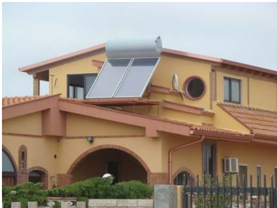
Solar-thermal installation on residential building
