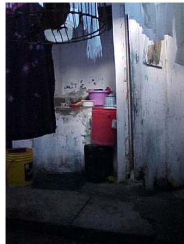
Humidity problems due to leaking roof structures.
