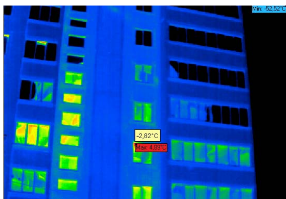
Photo made with thermal imager of the building on M. Dragan 38/2 str. and the neighboring building on M. Dragan 36/2 str. [IX]
