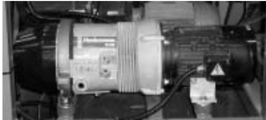
Figure 38: The compressor and the electric motor.
