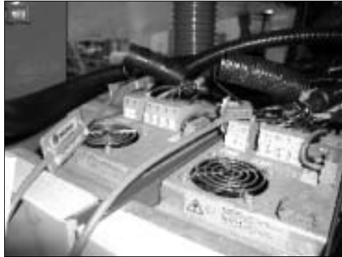
Figure A.4: The current sensor for the hydraulic pump, water-pump/air compressor
