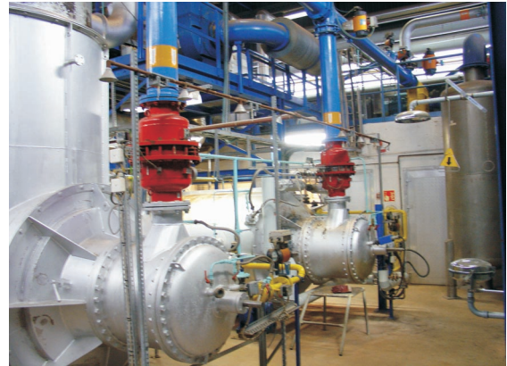
Fig. 2. An inside view of the incinerator hall. The photograph is taken from the position corresponding to the lower left corner of Fig. 1, showing the cyclone next to antenna position 5 at the rightmost of the picture.
