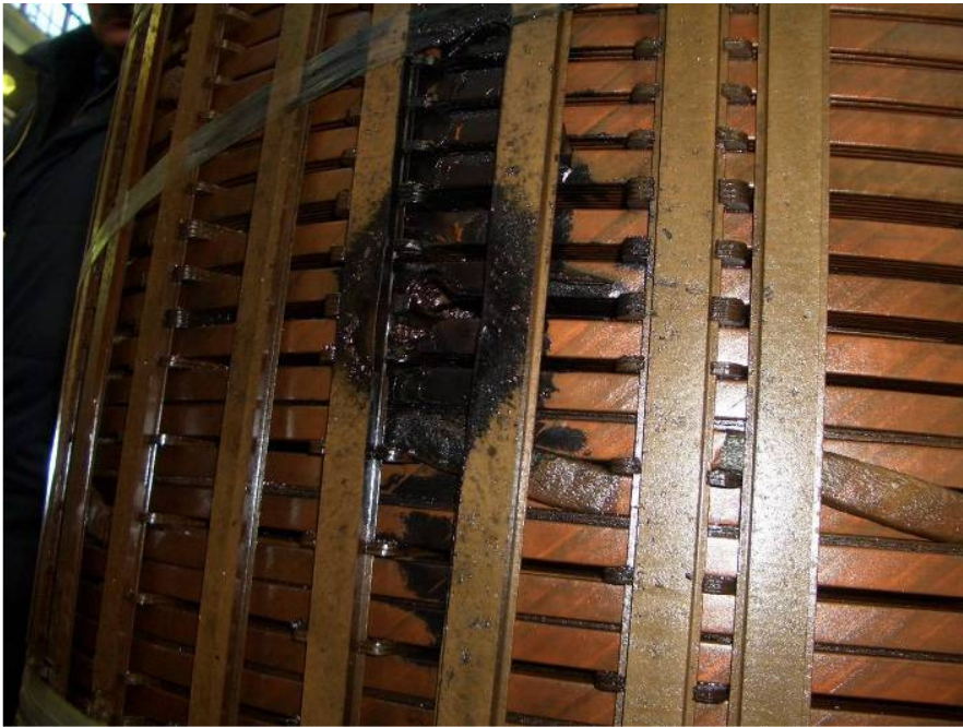
Figure 108: 35kV winding internal fault in phase L2.
