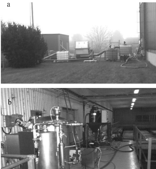
Figure 8 a,b) Pilot plant at Lundåkraverket WWTP, Landskrona, Sweden.
