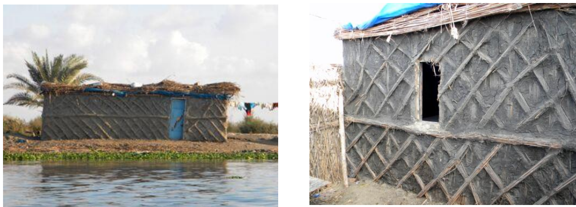
Fig (8) A crudely applied mud mortar (the mud of the lake is black, and making the hut appear dull grey when dry) –the dweller admitted that the quality of the hut and the plastering are not as good as they used to be since most of the few remaining huts are used as rest houses or shelters for fishermen.
