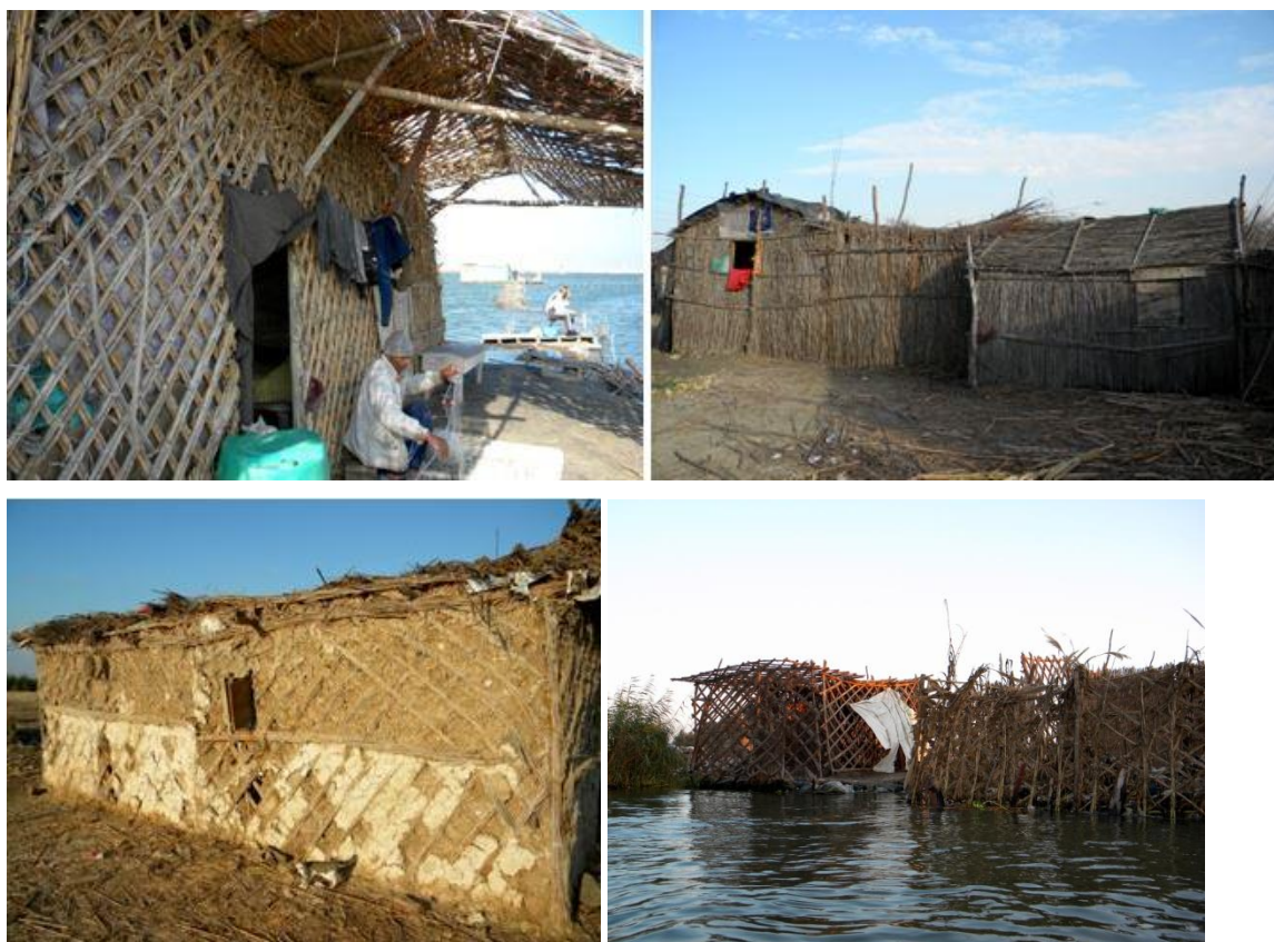
Fig (10) Examples of the dilapidated and poorly maintained remaining structures.
