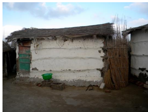
Fig (7) The dwellers added cement coats, especially at the base to create a plinth. Whitewashes are still applied to brighten the muddy surroundings.
