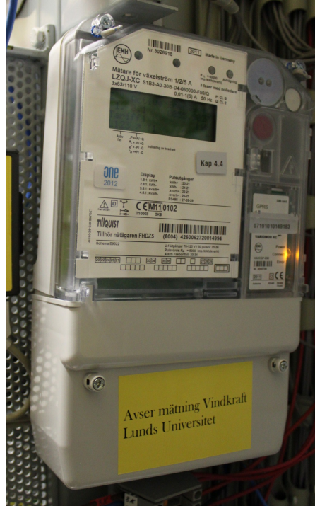
Figure 5.5: Electricity meter of type EMH LZQJ-XC which is mainly used in the field test.
