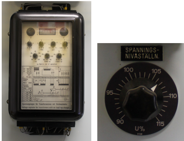
(a) Front panel of the AVC relay (b) Potentiometer to adjust AVC relay setpoint
